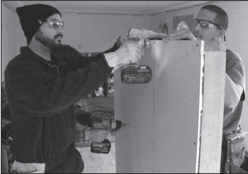
Student Bronson Gonzales, left, learns the finer points of drywalling from crew supervisor Manny Santos. Santos and AmericaCorps volunteer Tyler Ellifritz have directed the "pioneers" in a home remodeling project on East Sixth Avenue near Sheridan Elementary School.
